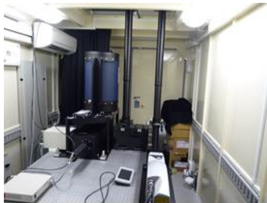
Fig.2 Mie lidar installed in the container.
