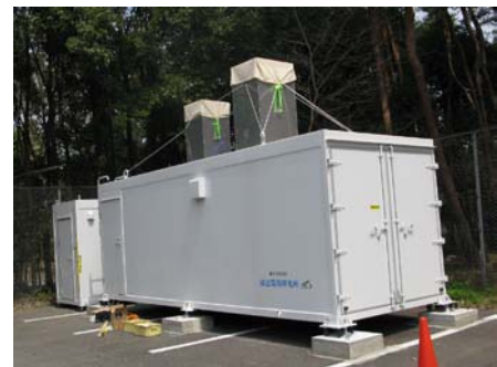
Fig.2 A container (front) and a chiller (back) for the mobile lidar.
