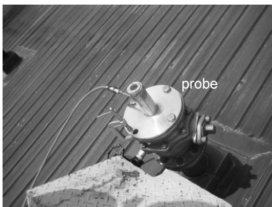
Fig. 6 Device with probe installed
