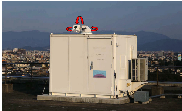
Fig. 2 Photograph of the 3D-CDL instrument installed at top of building A of Fukuoka University.
